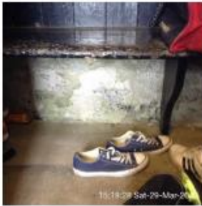
Poor state of repair
