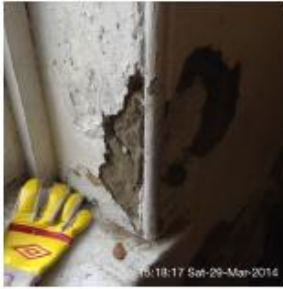
Poor state of repair
